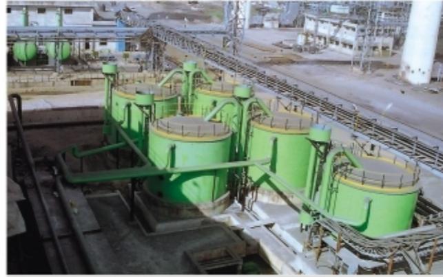
Part of water treatment system supplied to Bhushan Steel and Strips Limited
