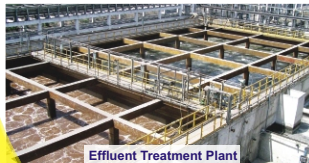
Effluent Treatment Plant
