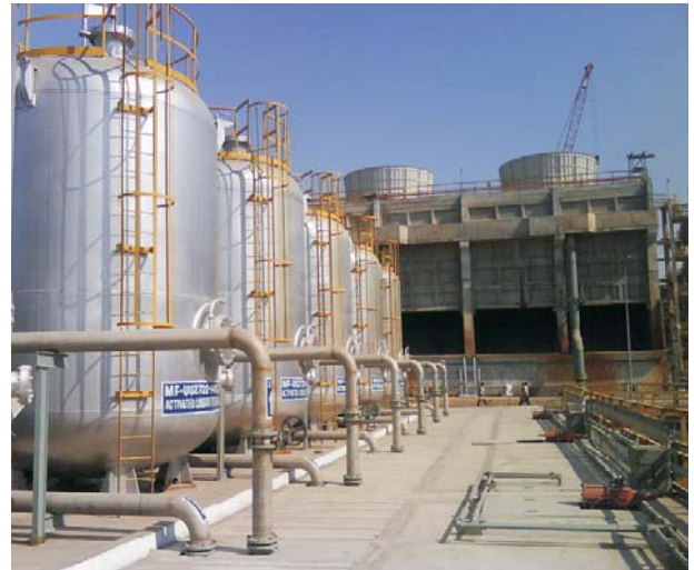
Activated carbon filters
