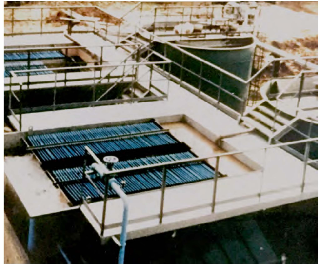
Installation in India of 2 x 100% lamella clarifiers with flocculation tanks. Each clarifier is rated for a maximum flow of 240 m 3 /h
