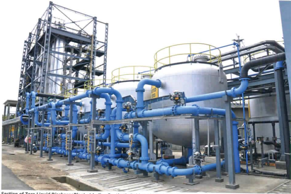
Section of Zero Liquid Discharge Plant at Indian Synthetic Rubber Limited
