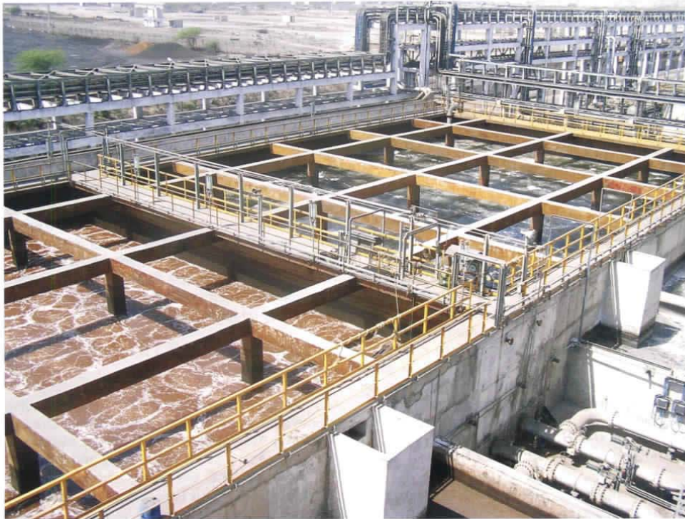
Effluent Treatment Plant at Reliance Industries Limited, Jamnagar, Gujarat
