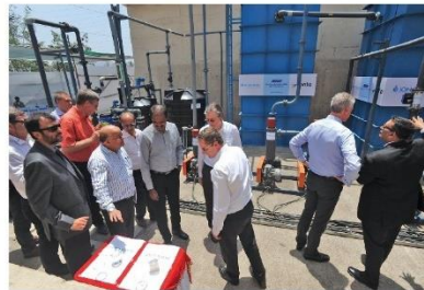
Installed as a pilot plant in India, the facility is being used as an alternate source of water at the Corporation's premises.
