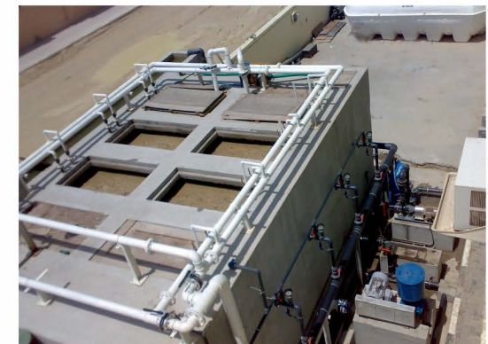
Membrane Bioreactor at Commercial Complex
