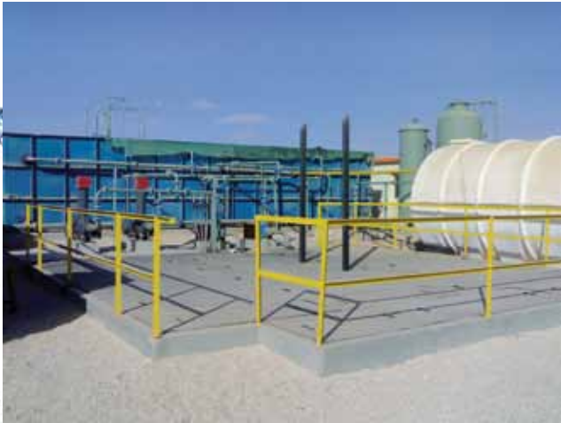
Packaged sewage treatment plant (200 m 3 /d fluidised media reactor) supplied to Gulf Petrochemicals Services & Trading (GPS) for the camp (1000 – 1200 people) located at Mukhaizna site where GPS was executing a project for Occidental Oman. The plant was delivered to site within three months and its erection and commissioning completed in 40 days
