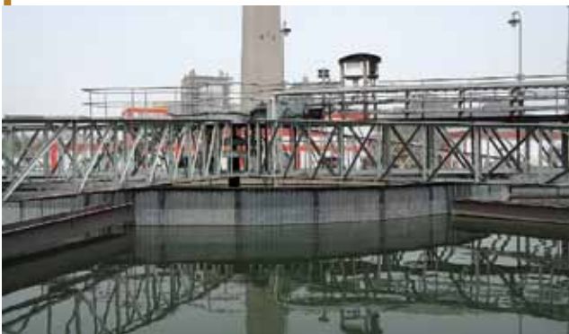
High rate solids contact clarifier
