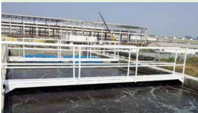
370 m 3 /d sewage treatment
