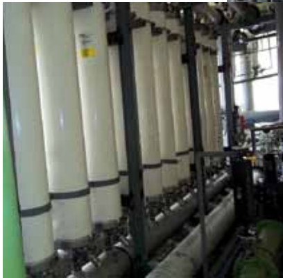
Ultra filtration stream
