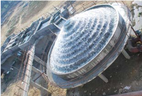
Pretreatment (cascade aeration)
