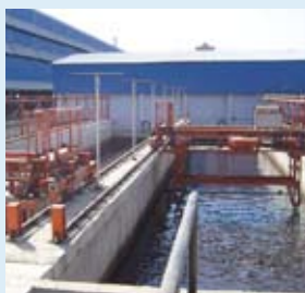
Settling tank with scraper mechanism
