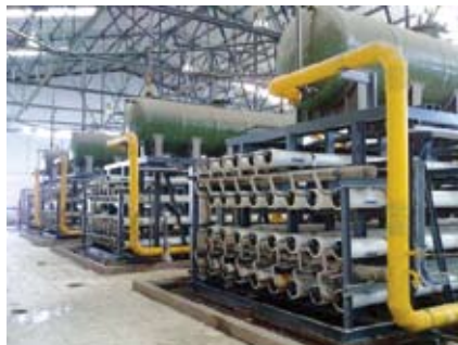
Reverse osmosis section
