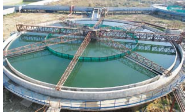
Pretreatment (high rate solids contact clarifiers)
