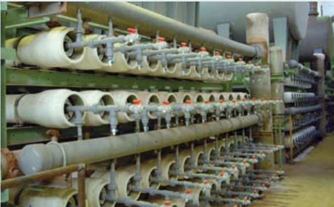
Reverse osmosis section
