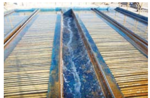
734 m 3 /h lamella clarifier
