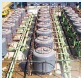
Pressure filtration plant
