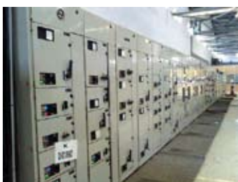
Primary motor control centre (PMCC)
