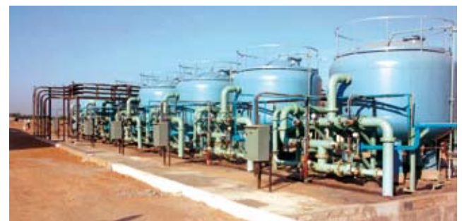
Pressure sand filters
