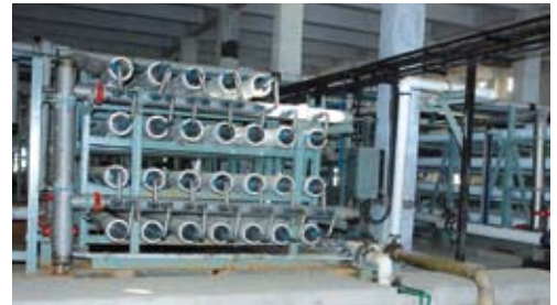
Reverse osmosis section
