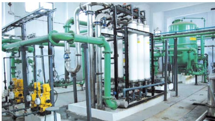
Ultra filtration section
