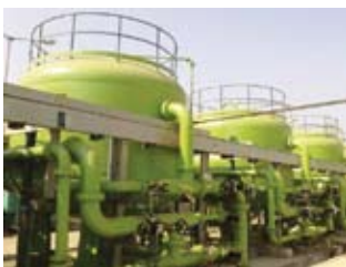
Pressure sand filters
