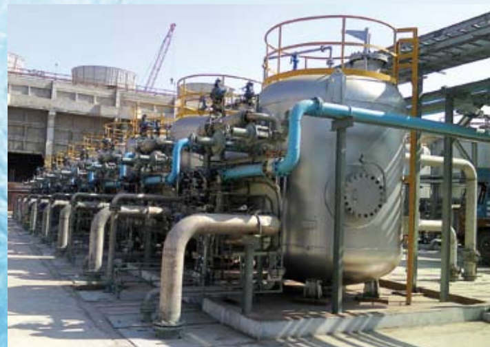
Condensate polishing plant
