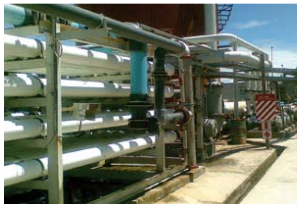
Commissioned for a copper mining company in Zambia, Africa, water treatment plant, 1000 m 3 /h pretreatment and 3x175 m 3 /h RO.
