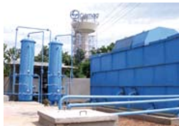
At L & T Demag, Chennai, 35 m 3 /day NGPSTP
