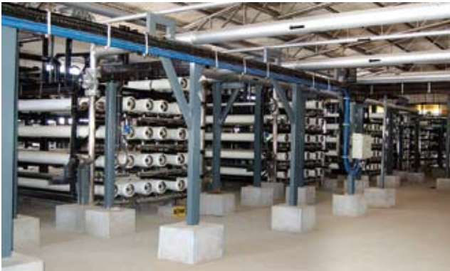
Reverse osmosis section
