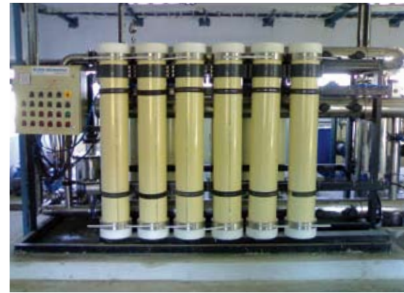
Ultra filtration section
