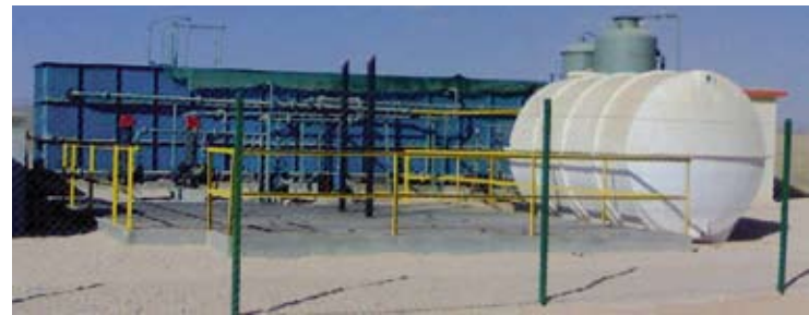
Fluidised media reactor
