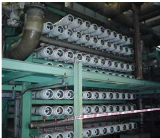
Reverse osmosis section
