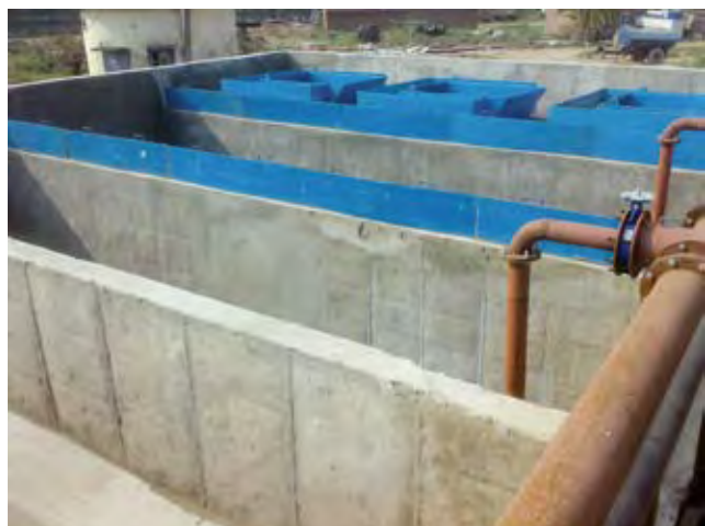
1000 m 3 /d fluidised media reactor (FMR) at MES (Civil), Pathankot, Punjab
