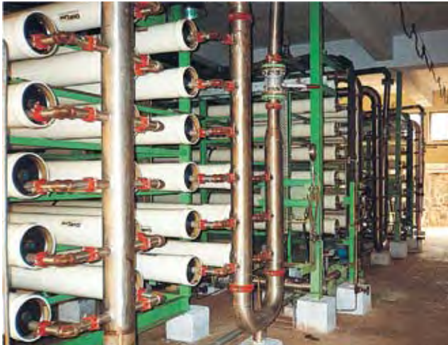
Zero discharge plant
