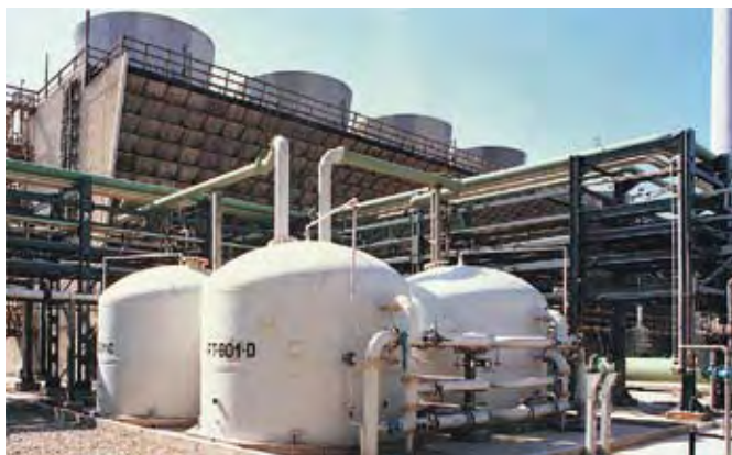
Cooling water treatment
