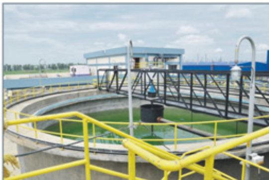
High rate solids contact clarifier
