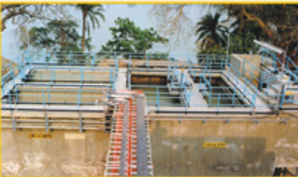
Drinking water treatment for a municipal corporation
