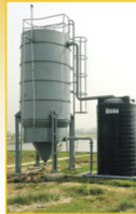
Continuous sand filter for surface water treatment
