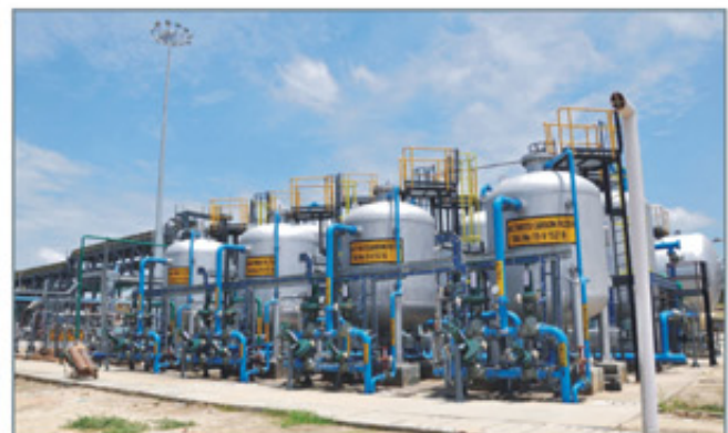
Activated carbon filters
