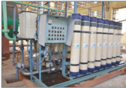
Ultra filtration plant
