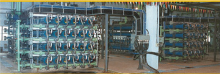
SWRO plant at GEB, Sikka
