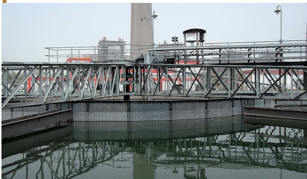
High rate solids contact clarifier
