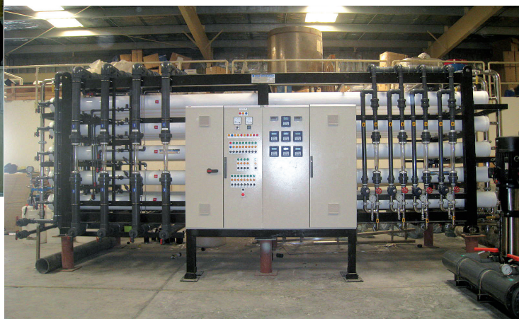
Four stream reverse osmosis plant of 3850 m 3 /day, supplied to Petroleum Development of Oman (PDO) at Faud site, Sultanate of Oman
