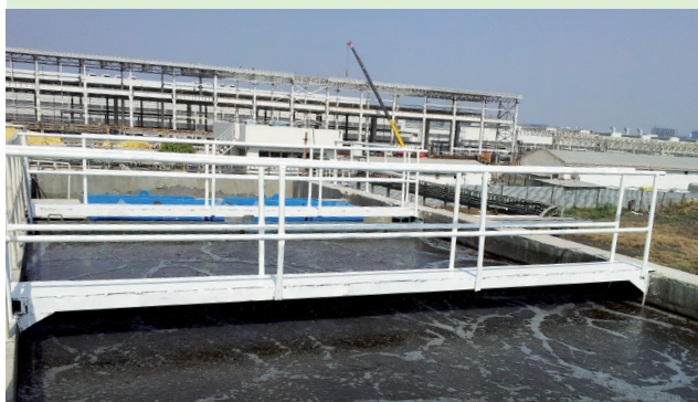
370 m 3 /d sewage treatment
