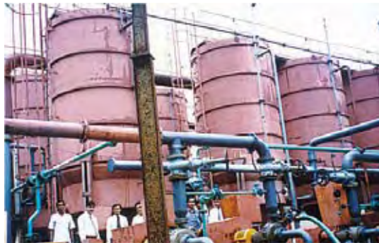
Continuous sand filters for white water recycle in paper mill
