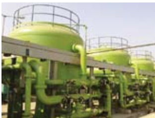
Pressure sand filters
