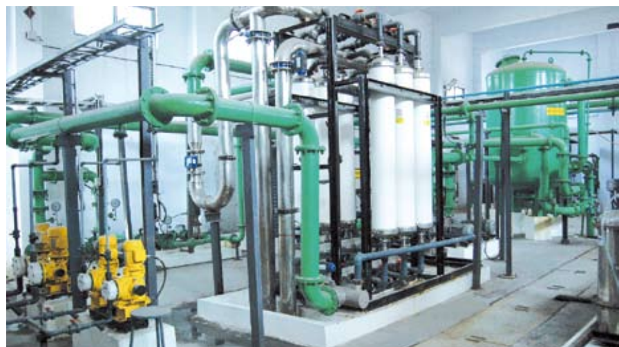
Ultra filtration section
