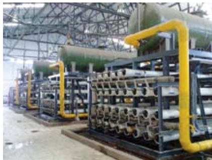
Reverse osmosis section
