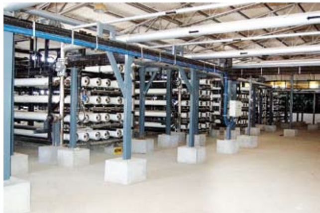
Reverse osmosis section
