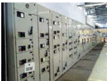
Primary motor control centre (PMCC)
