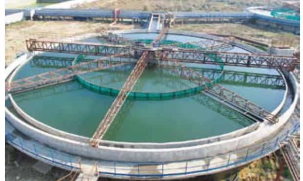
Pretreatment (high rate solids contact clarifiers)
