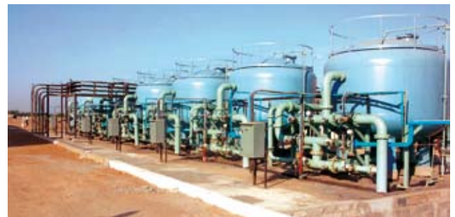
Pressure sand filters
