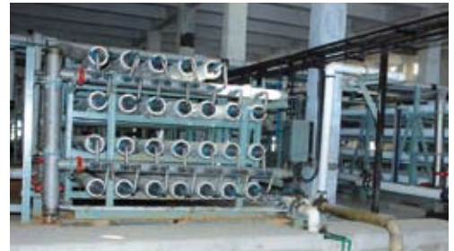
Reverse osmosis section
