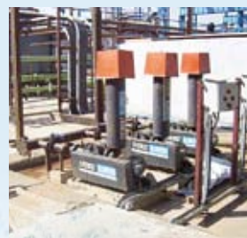
Air blower for pressure filtration plant
