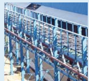
Overhead pipe trestle plant
