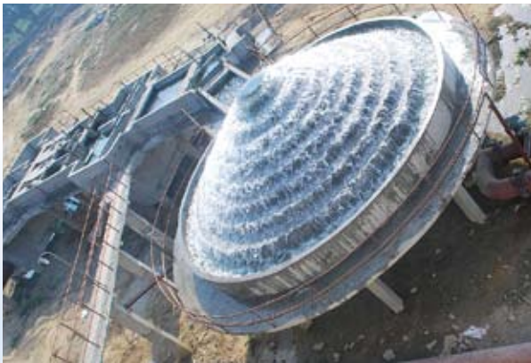
Pretreatment (cascade aeration)
