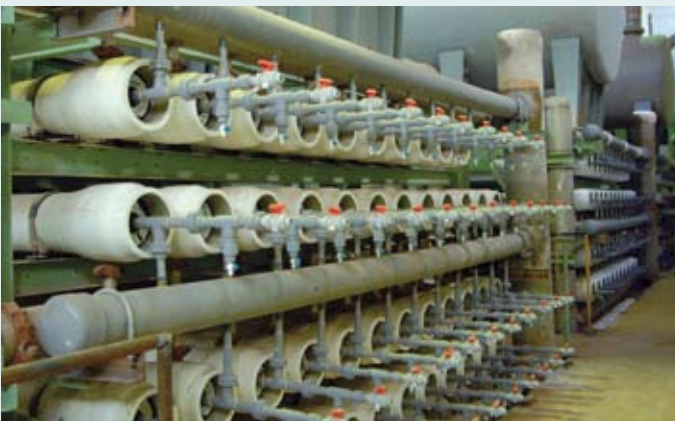
Reverse osmosis section
