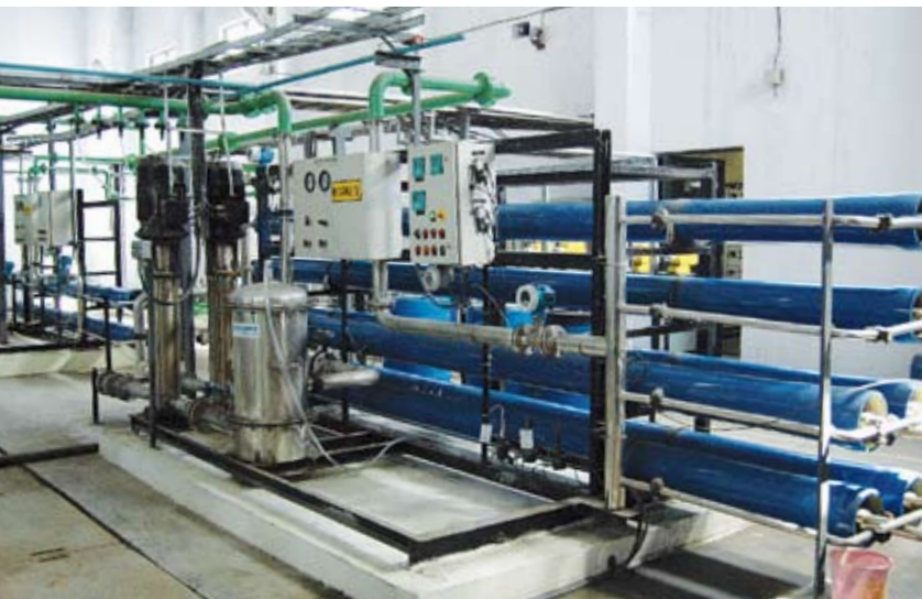
Reverse osmosis section
