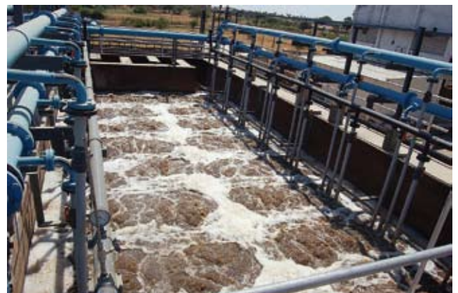
Membrane bio-reactor section
