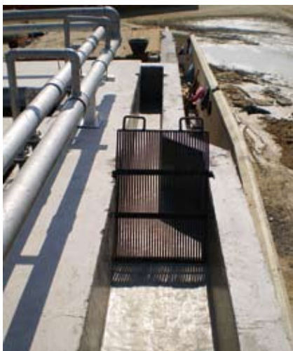
Membrane bio-reactor section
