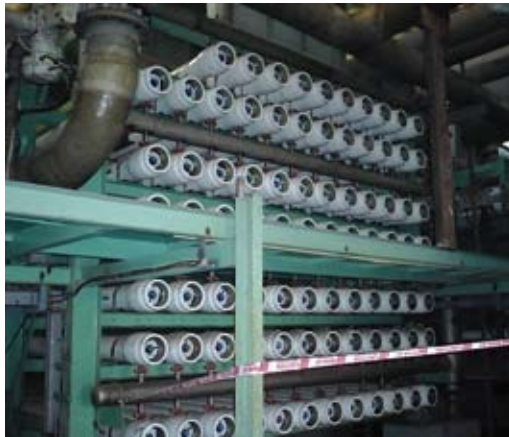
Reverse osmosis section
