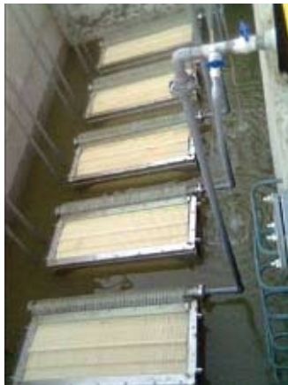
Membrane bio-reactor section
