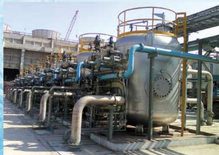
Condensate polishing plant
