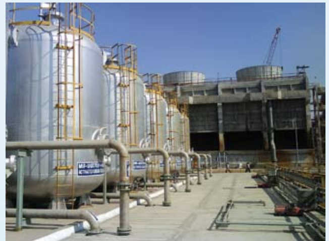
Activated carbon filters
