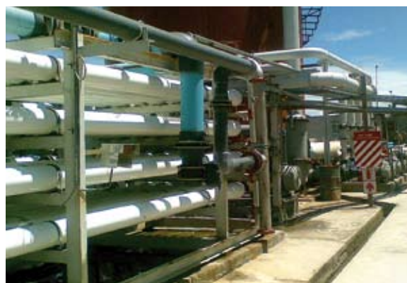
Commissioned for a copper mining company in Zambia, Africa, water treatment plant, 1000 m 3 /h pretreatment and 3x175 m 3 /h RO.
