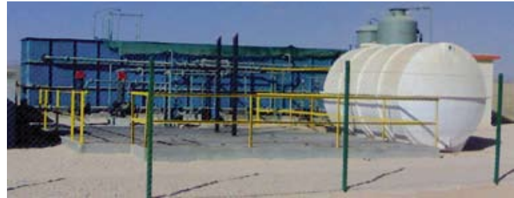
Fluidised media reactor
