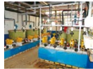
Effluent Treatment Plant
