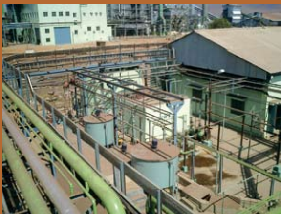
Water treatment plant (high rate solids contact clarifier, ultra filtration, reverse osmosis and demineralisation) commissioned at BMM Ispat, Hospet, Karnataka.
