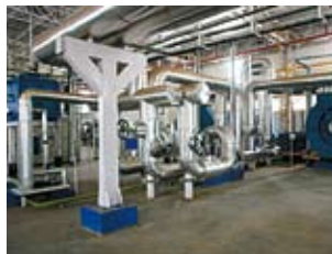
Hot Water Generators
