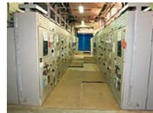
Motor Control Centre
