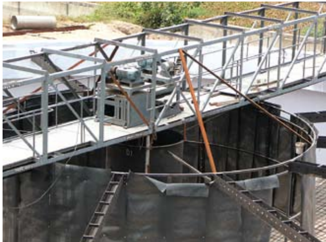
High Rate Solids Contact Clarifier
