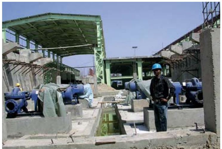
Indirect Cooling Water Pump House
