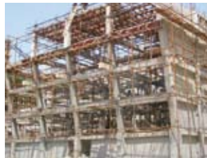
Direct Cooling Water CT
