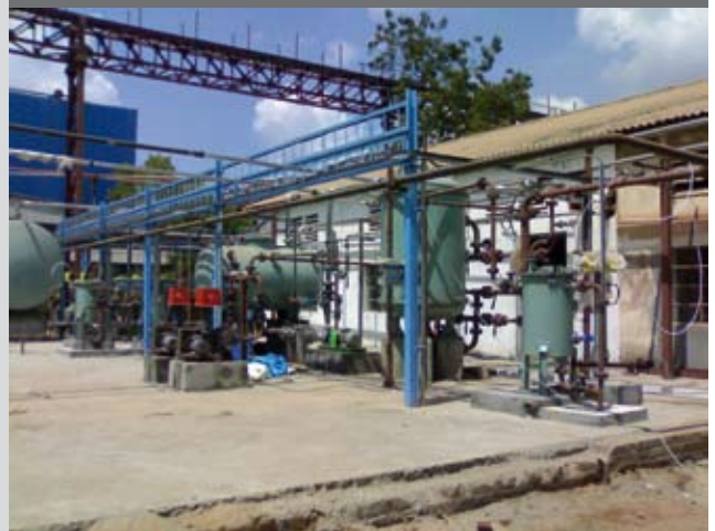
Water treatment plant for Chettinad Cement Corporation, Puliur, Tamil Nadu. The scheme includes pressure sand filtration, ultra filtration, reverse osmosis, degassification and demineralisation.
