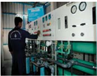
Operating RO plant at O&M site
