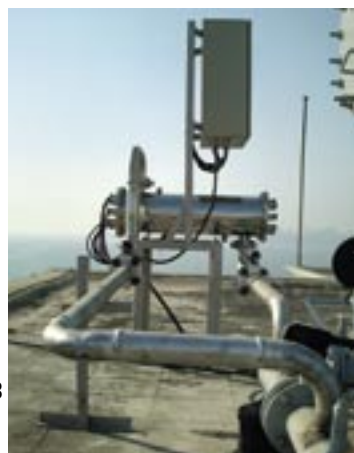
At Hotel Marine Plaza, Mumbai modification of 15,000 LPH UV system with GI pipeline.
