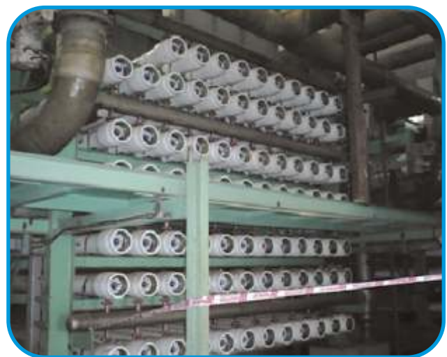
Reverse Osmosis Section
