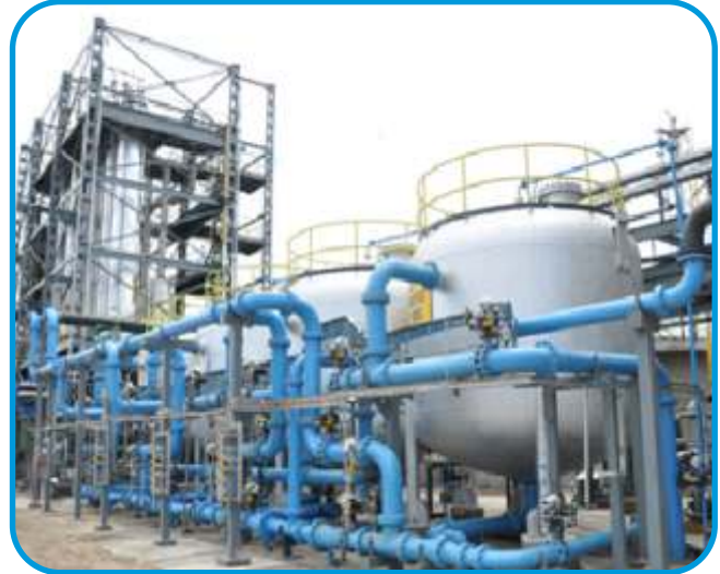
Complete Zero Liquid Discharge
