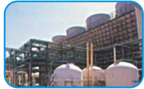
Indion Cooling Water Treatment Programme
