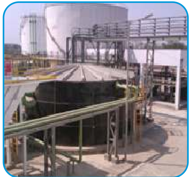
Indion Zero Liquid Discharge
