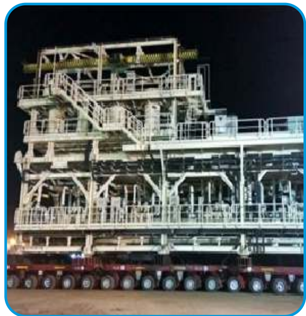
Complete assembled skid being moved on Self Propelled Modular Transporter (SPMT) from Fabrication Yard to Barge
