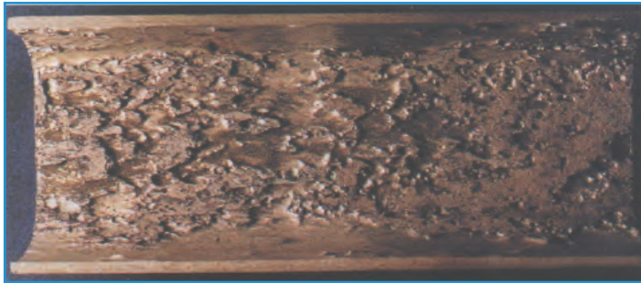
Fig 10.7 - Photograph of boiler tubes with deposits
