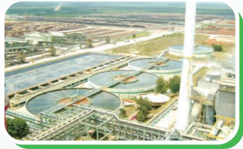
Clarifiers section at a paper plant
