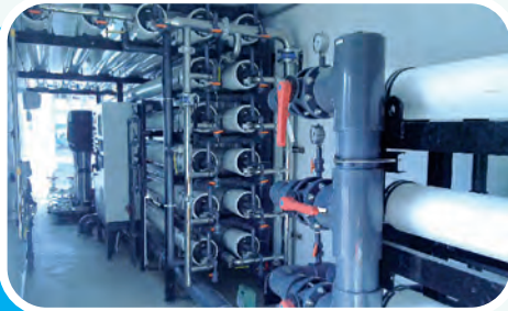
Brackish water reverse osmosis unit at a power plant
