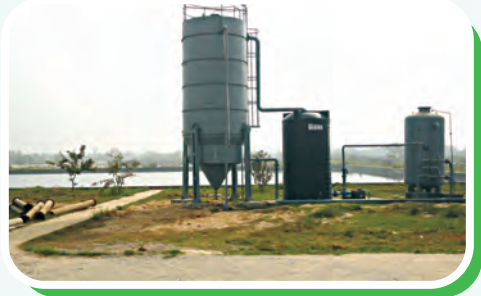
Continuous sand filter for surface water treatment
