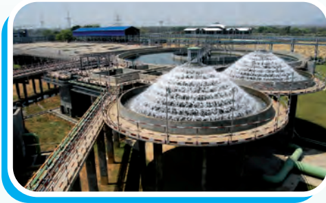
Cascade aeration at a power plant
