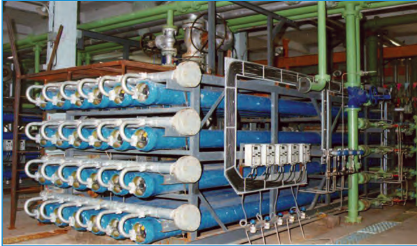
Fig 11.7 - Photograph of fully assembled RO skid
