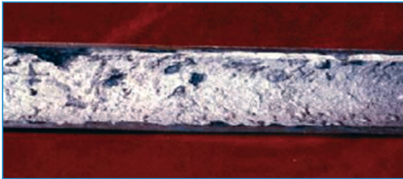
Fig 10.6 – Photograph of severely scaled boiler tube
