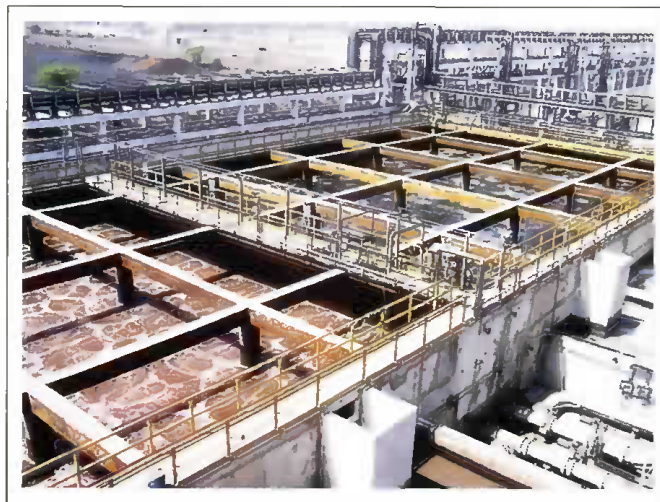
Effluent Treatment Plant at Reliance Industries Ltd., Jamnagar, Gujarat
