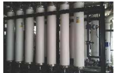
Ultra Filtration Plant
