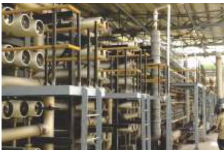
Reverse Osmosis Plant
