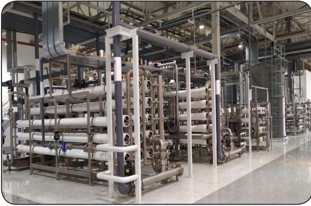
Zero Liquid Discharge System for a major Multinational Automobile manufacturer
