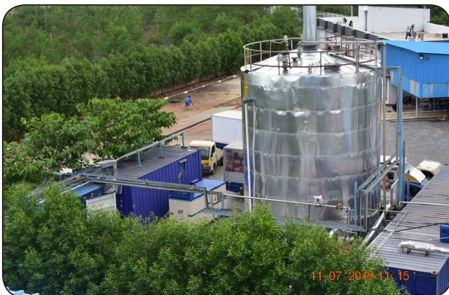
ANDICOS Waste to Energy Plant
