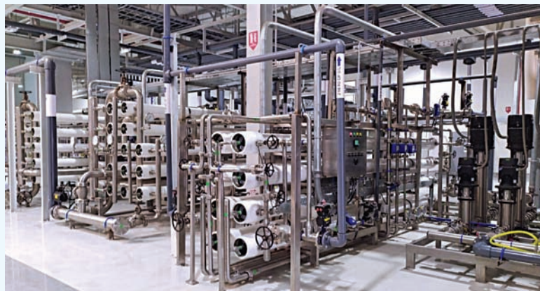
Total Water Management with Zero Liquid Discharge System for a major multinational Automobile manufacturer
