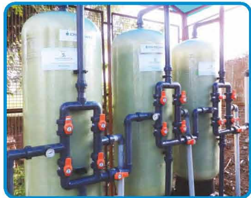
INDION Arsenic Removal Tubewell Attachment at Kuralita Village, Punjab for Providing Safe Drinking Water to the Villagers
