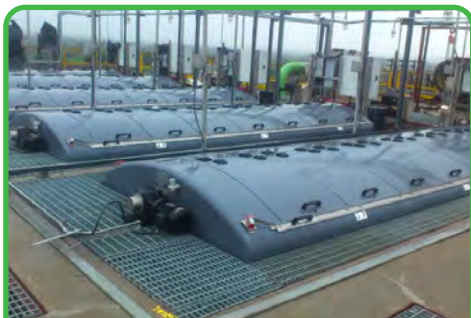
Advanced Sewage Recycle Systems
