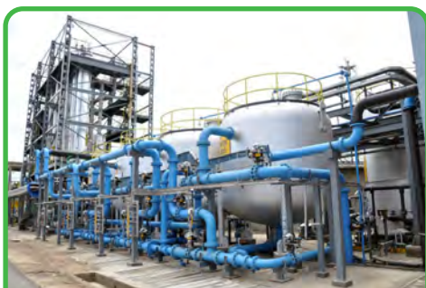
Complete Zero Liquid Discharge
