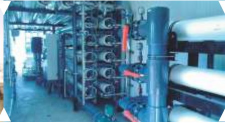
Desalination Plant for Al Ghubrah Power, Oman
