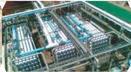
Reverse Osmosis System for Vedanta Group, Konkola Copper Mines, Zambia, Africa
