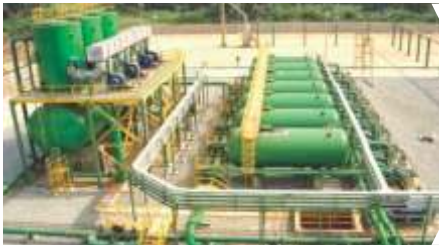
Pretreatment at OKPAI Power Plant, Nigeria
