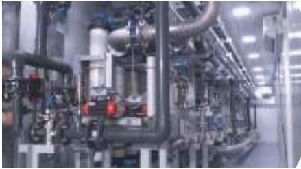
ETP Plant with containerised UF System for Air Liquide Global E&C Solutions
