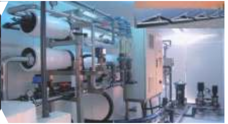
Solar Powered Sea Water Reverse Osmosis for a Tourist Development Complex, Abu Dhabi
