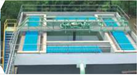
Ultra High Rate Clarifier at PT South Pacific Viscose, Indonesia
