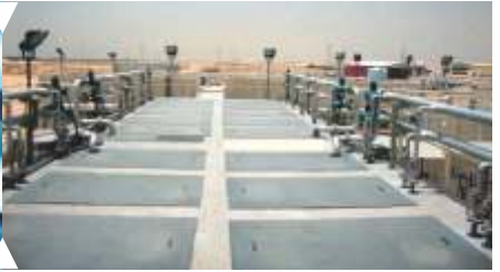
Membrane Bio-reactor Plant at Industrial Area, UAE
